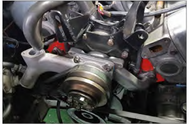
NEW PUMP IN SITU
